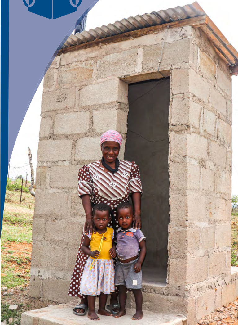
Tfobhi Simelane, with her grandchildren, standing in front of her newly constructed toilet, built by members of the community through the food-for-asset project.
